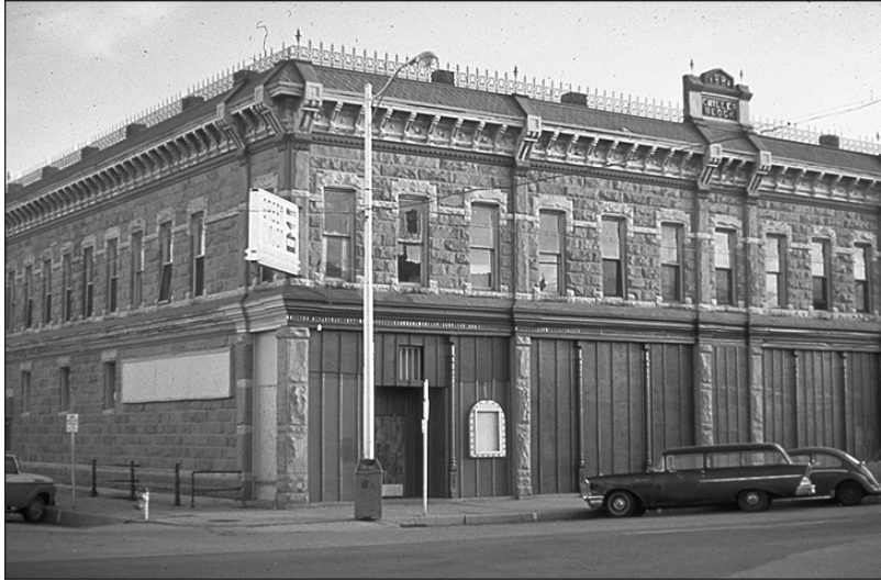
In the early 1980s, the windows in the Miller Block were boarded and architectural details needed repair.
