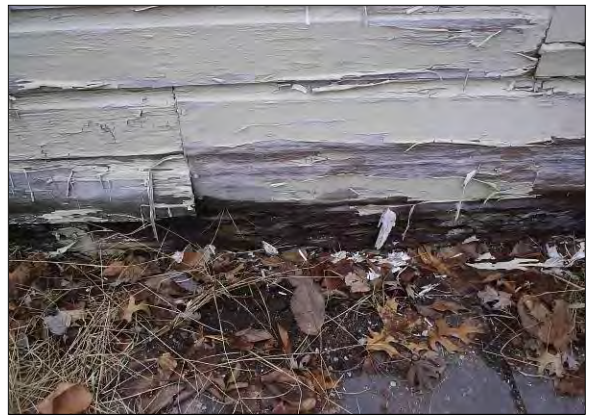
Peeling Paint, Wood at bottom is rotting
