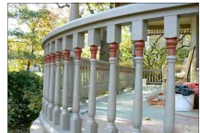
Original balusters are repaired and repainted retaining the original material and integrity
