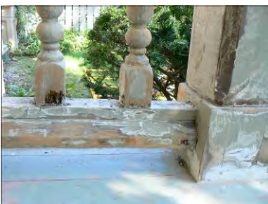
Paint stripped from balusters and some decay is found
