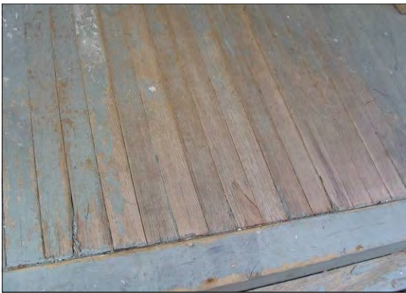
Worn Paint, Wood in good condition
