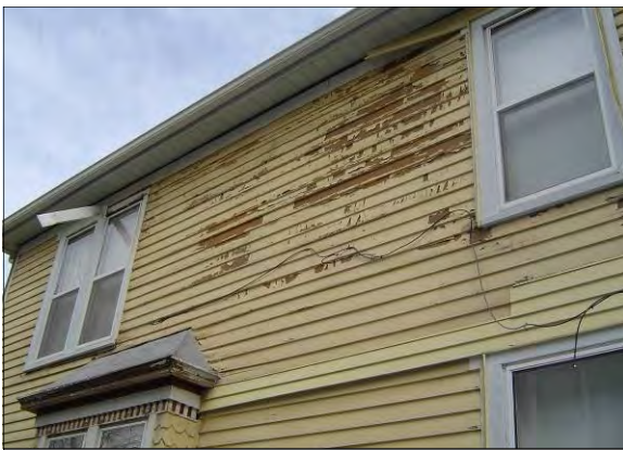
Peeling Paint, Wood likely in good condition
