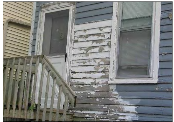
Peeling Paint, Wood may be in bad condition
