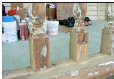
Small decay holes filled with epoxy, larger ones replaced with new wood
