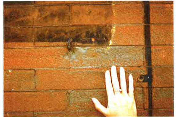
Sandblasting removed the outer surface of this brickwork, exposing the soft interior to water penetration and subsequent freezing and thawing damage.
