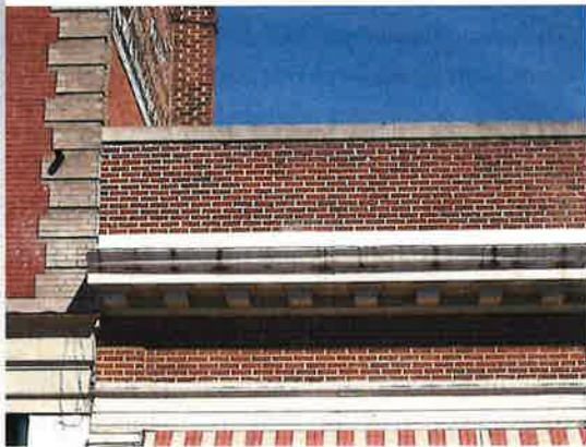
This roof should retain its flat pitch if rehabilitation or other alterations are undertaken on the building.
