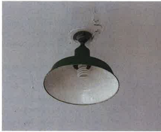
The placement and design of this modern lighting fixture are inconspicuous and non damaging to major building features. Additionally, the compact fluorescent light bulb in this fixture uses substantially less energy than a traditional incandescent bulb.
